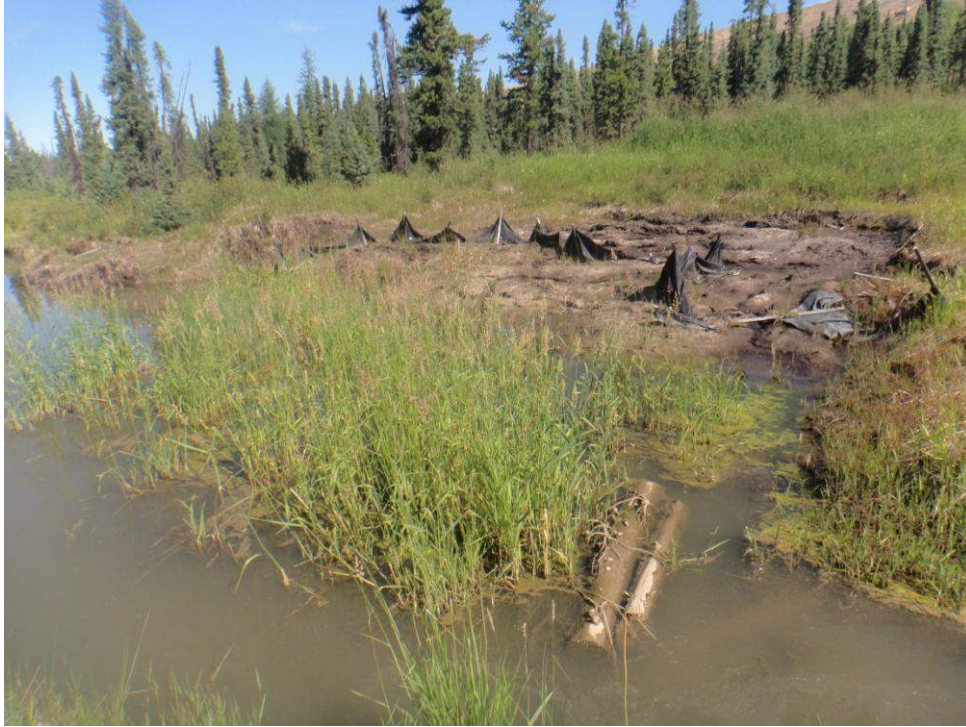
Photo 3. Erosion along lower end of Mercoal diversion channel (from Right Upstream Bank).
