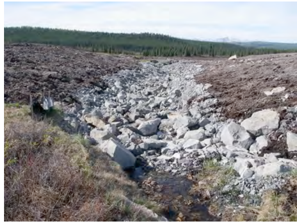
Photo 2. Looking downstream at restored channel from MET-3. Note: lack of surface connection
