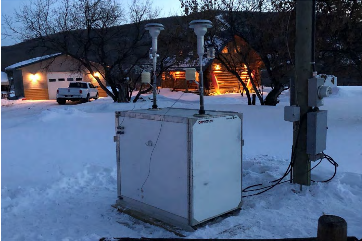
Figure 2-2: Upgraded Station 8 (Old Fort) with climate-controlled enclosure
