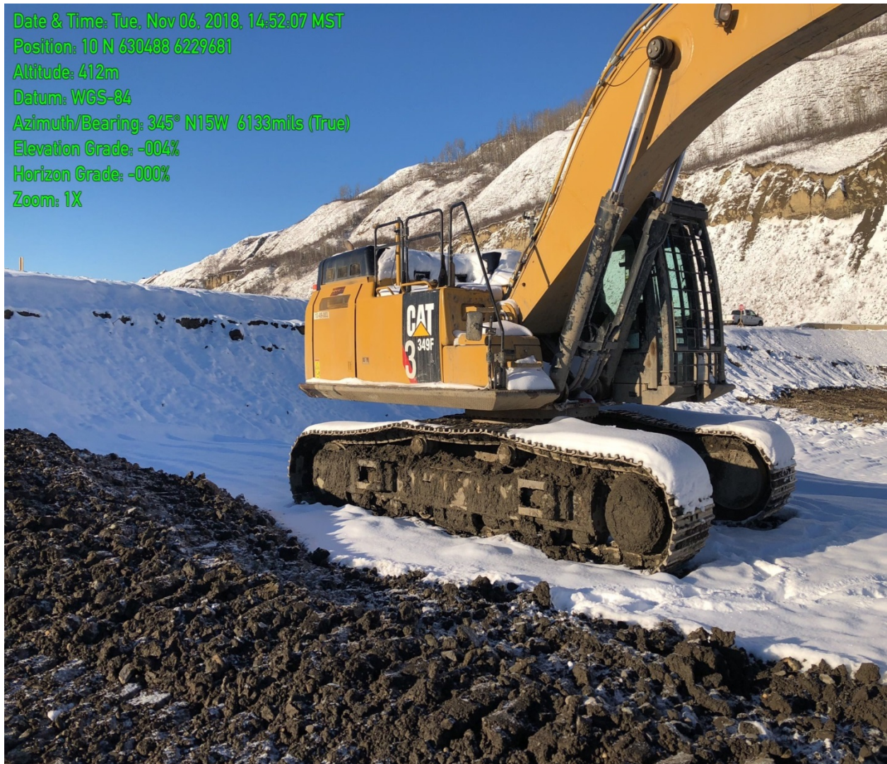
Figure 3. Biodegradable hydraulic fluids were used in equipment working above or within wetted areas during the construction of RSEM L6 (November 6, 2018).
