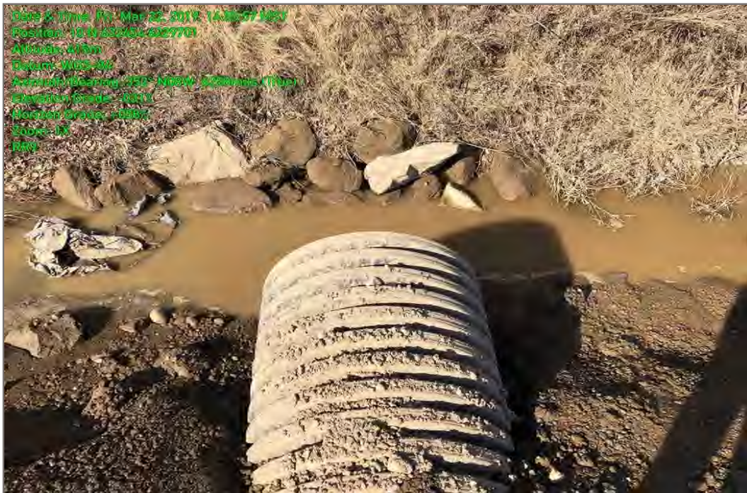
Photo 24: River Road water sample location RR9 at culvert inlet, dated March 22, 2019.
