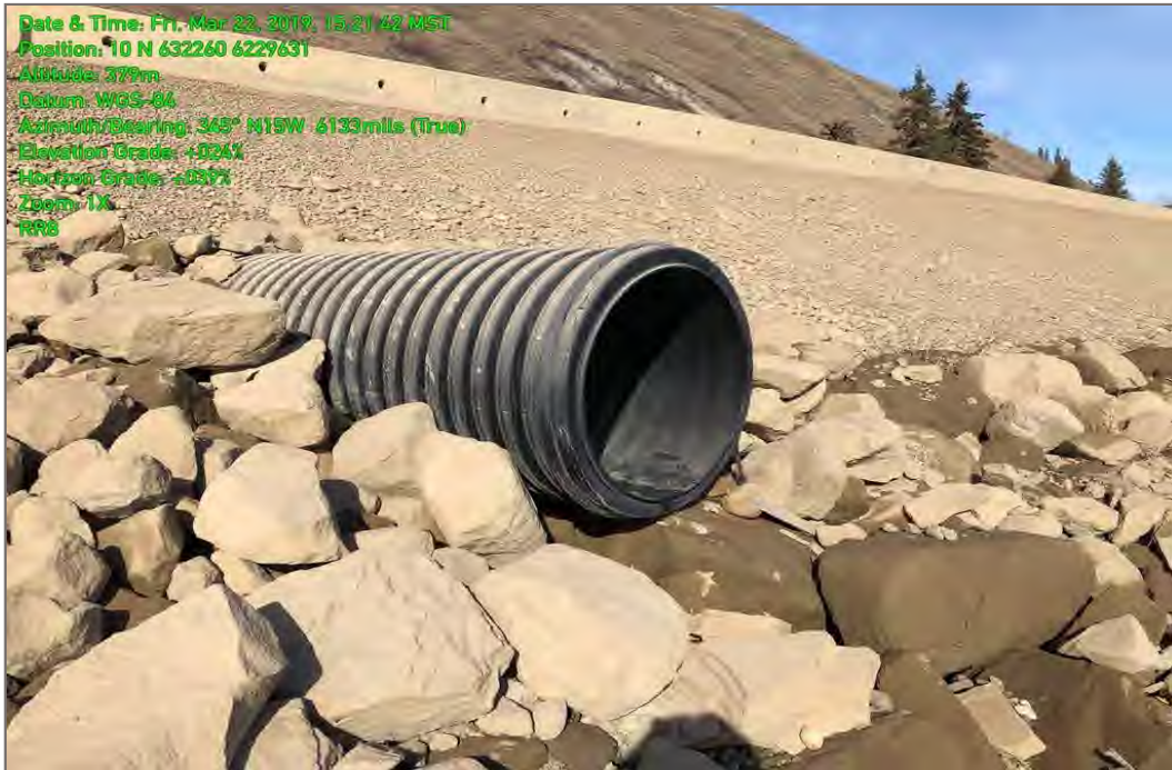
Photo 23: River Road culvert from RR8; no water flow; not a sample location, dated March 22, 2019.
