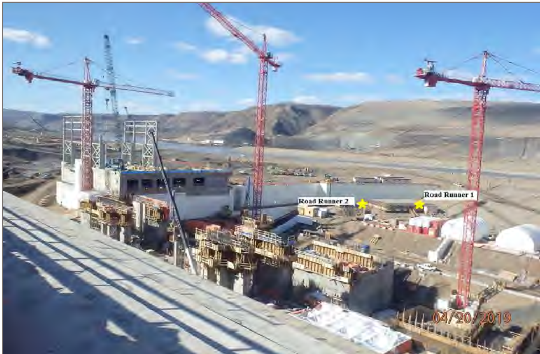
Photo 29: Road Runner 1 and Road Runner 2 water sample locations looking north, dated April 18, 2019.
