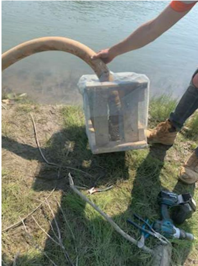
Figure 1. Addition of fish screen in accordance with DFO guidelines at Cache Creek Highway 29 realignment water withdrawal (July 14, 2021).
