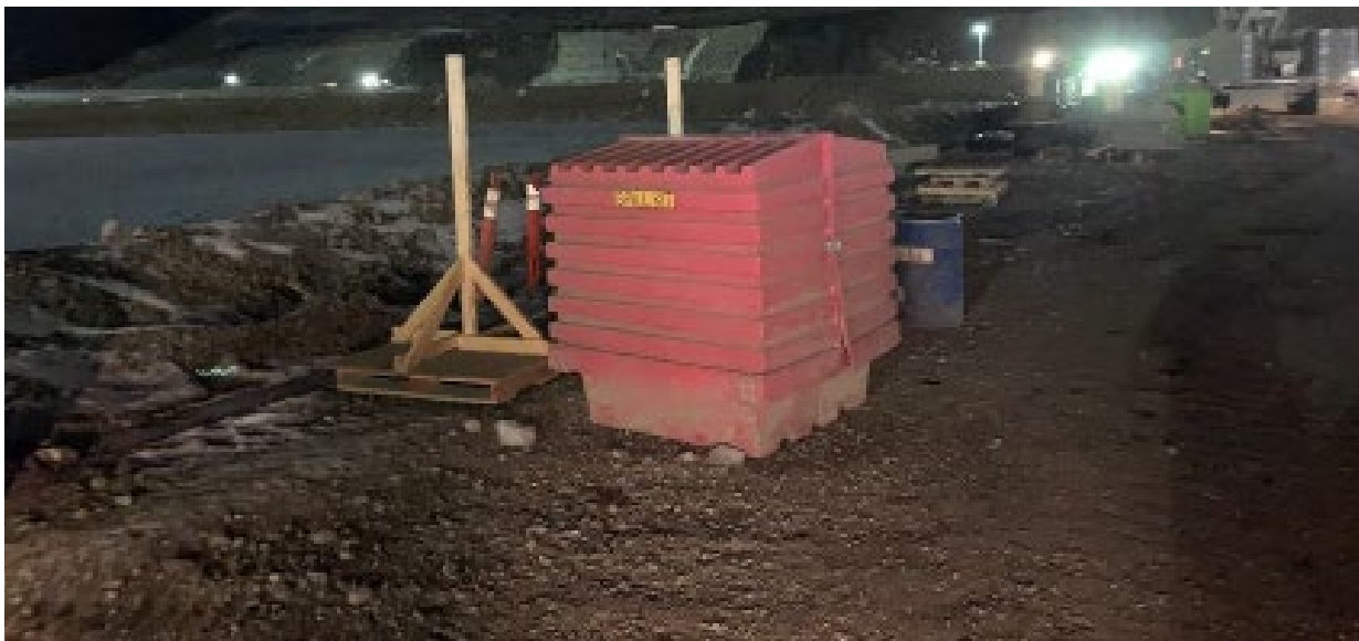
Figure 3. Spill prevention measures, including floating boom, within the dam site construction area adjacent to the Peace River (January 18, 2021).
