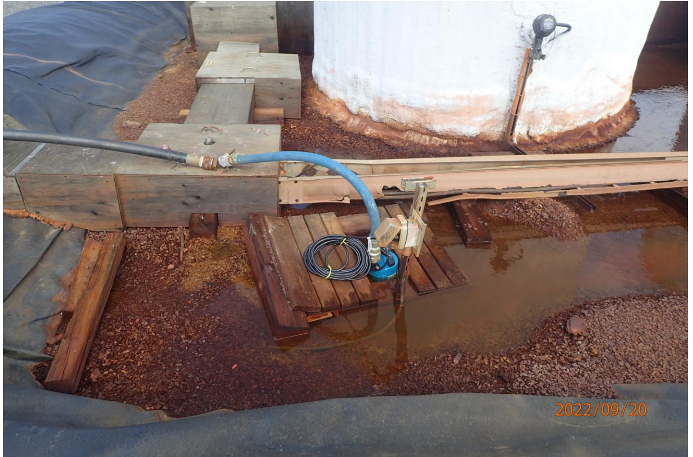
Photo 3: pump found dismantled at time of inspection
