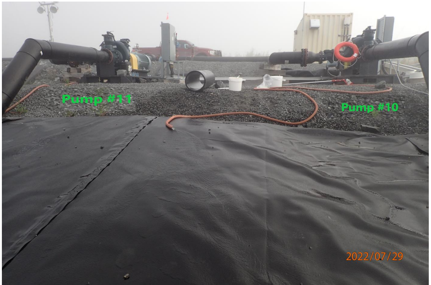
Photo 2: Outflow Basin Pumps
