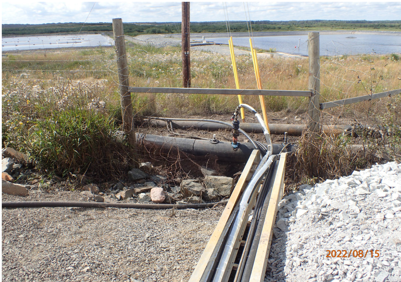
Photo 2: Spill location after clean up
