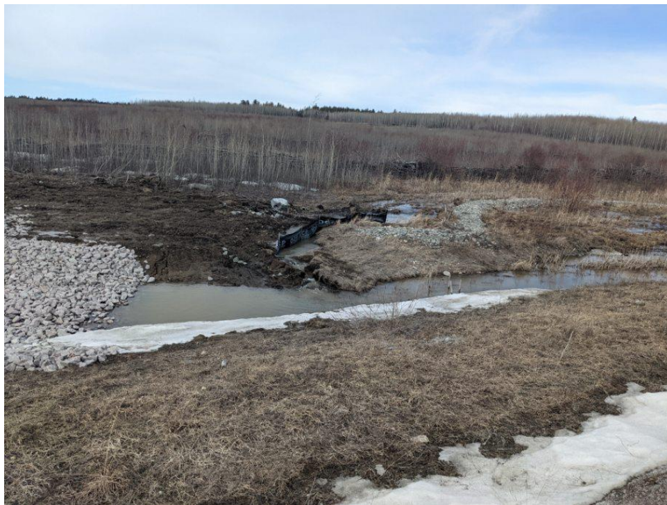
Figure 3 Inadequate sediment and erosion control measures at recently constructed TMA seepage pond.
