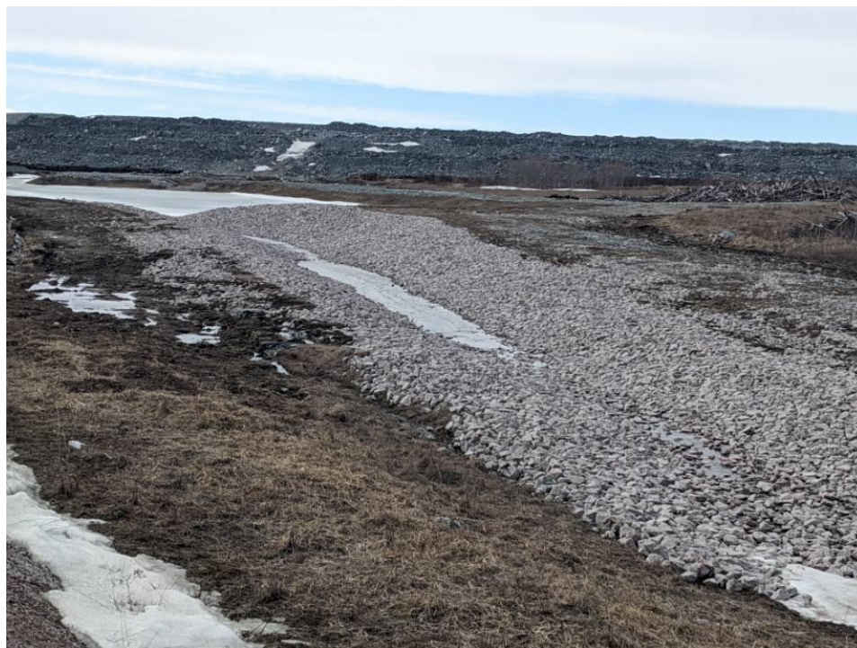
Figure 4 TMA seepage pond spillway activated.
