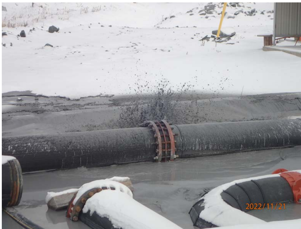
Photo 1: Leak at pipe connection
