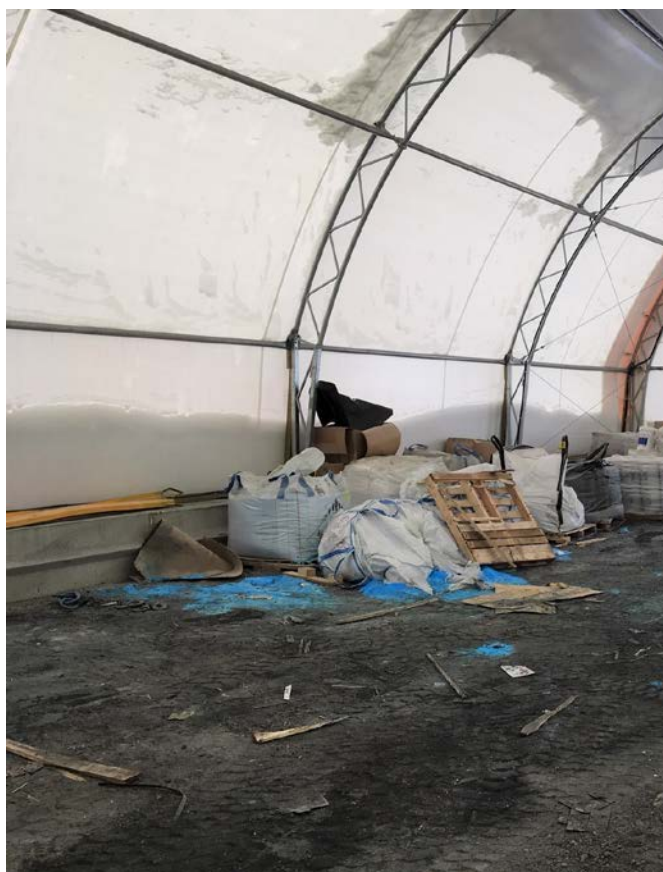
Figure 1: Location of copper sulfate spill inside the covered chemical cold storage building east of the Mill
