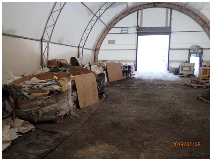
Figure 3: Cleaned up copper sulfate spill inside the covered chemical cold storage building east of the Mill. Damaged totes placed on fold out spill containment.
