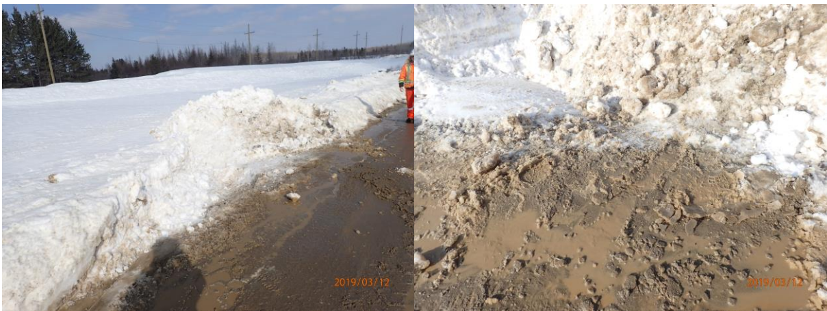
Figure 3. Punch out created on north side of Roen Road (left). Small swale made with shovel to help promote water-shedding from Roen Road (right).
