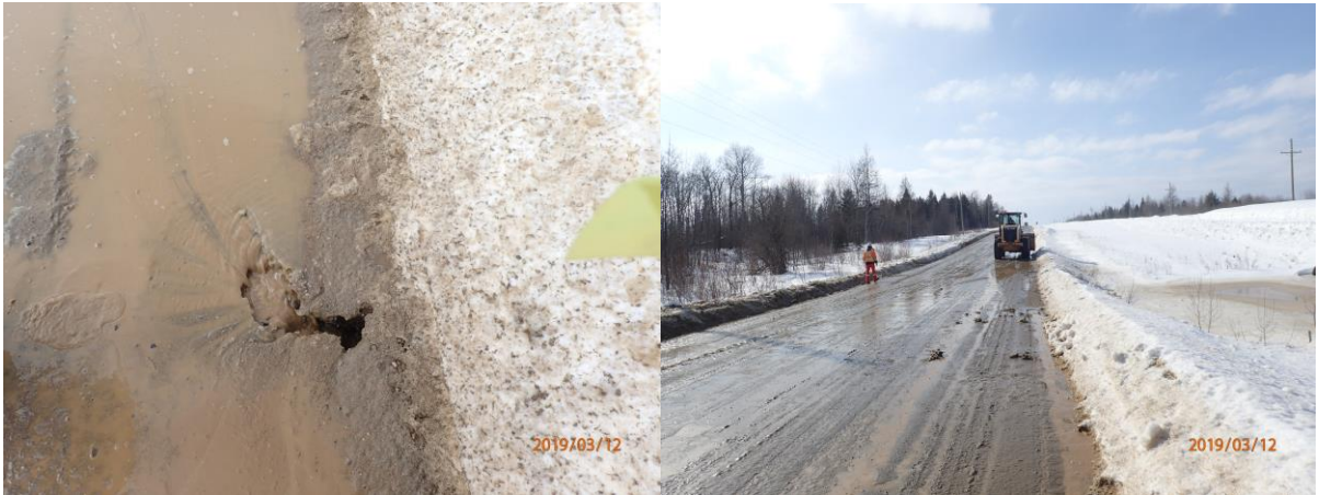
Figure 2. Eroded hole in Roen Road allowing turbid water from road to enter West Creek (left). Condition of road when mitigation measures were being installed by loader (right).
