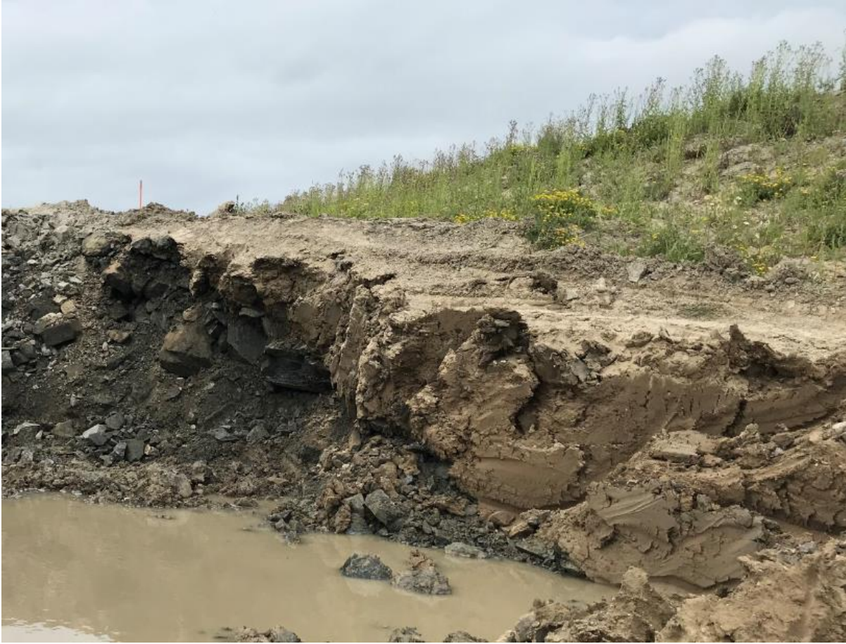
Photograph A.11: Borrow investigation of clay key layer on southeast corner of Trial #2. July 15, 2019.
