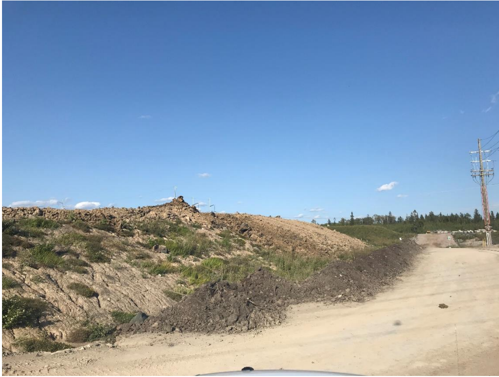
Figure 5: Construction in progress of the south slope of the vegetation trial landform.
