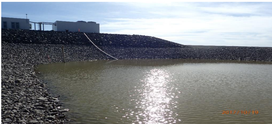
Figure 2: Water Management Pond Intake Structure, October 2017
