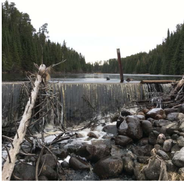
Figure 28. Dam at the downstream end of the Tree Nursery ponds on Thunder Lake Tributary 3. April 24, 2017.
