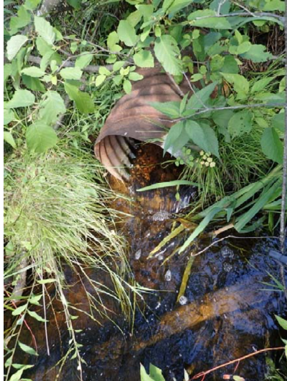
Figure 19. Corrugated steel pipe conveying Blackwater Creek Tributary 2 beneath a forestry road approximately 1.25 km upstream from Normans Road.
