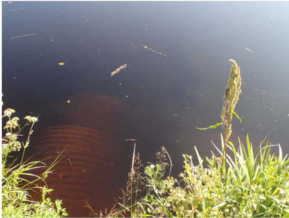
Figure 7. Upstream end of culverts underneath the railway that convey water from Blackwater Creek into Keplyn's Bay. August 3, 2016.
