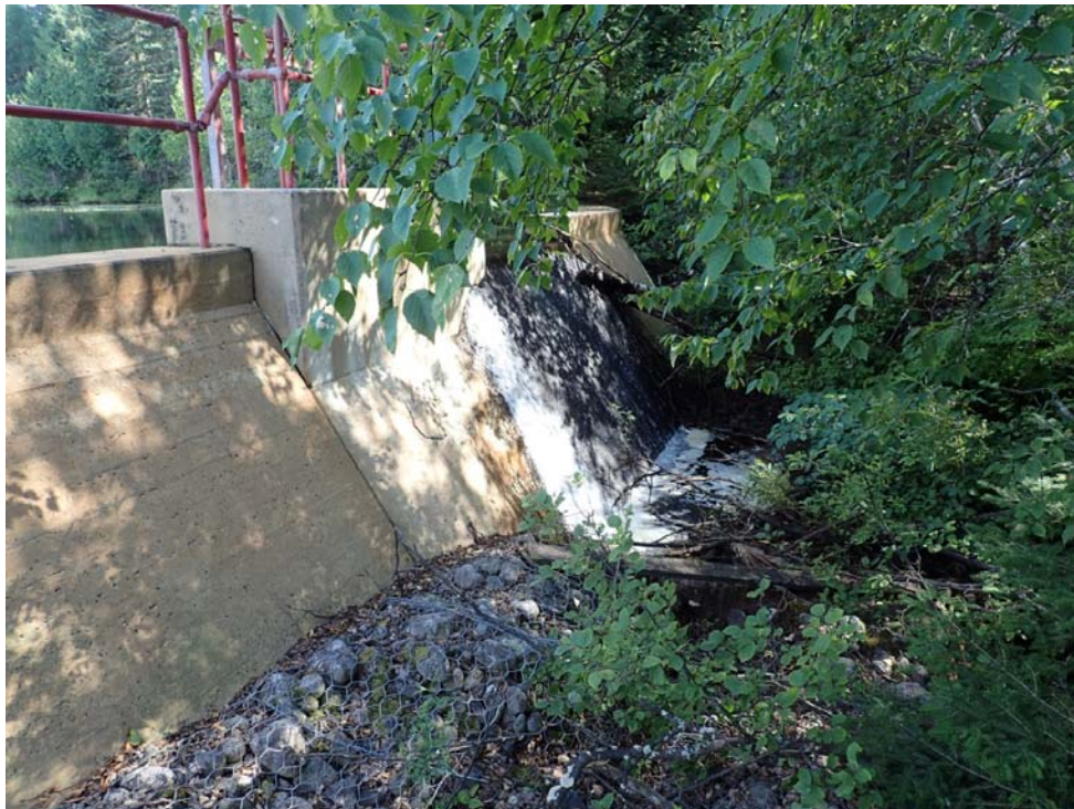
Figure 26. Dam at at the downstream end of the tree nursery ponds on Thunder Lake Tributary 2. August 3, 2016.
