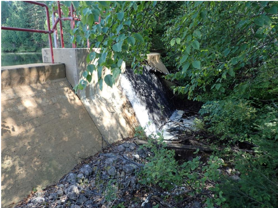
Figure 26. Dam at the downstream end of the tree nursery ponds on Thunder Lake Tributary 2. August 3, 2016.
