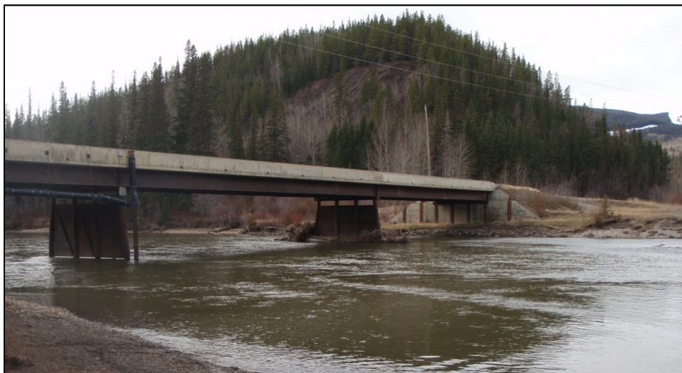
Plate 7.1-2. Murray River: view upstream at the Murray River FSR Bridge. Flow rate = 53 m 3 /s. A public access boat launch area is located adjacent to the bridge. April 28, 2012.
