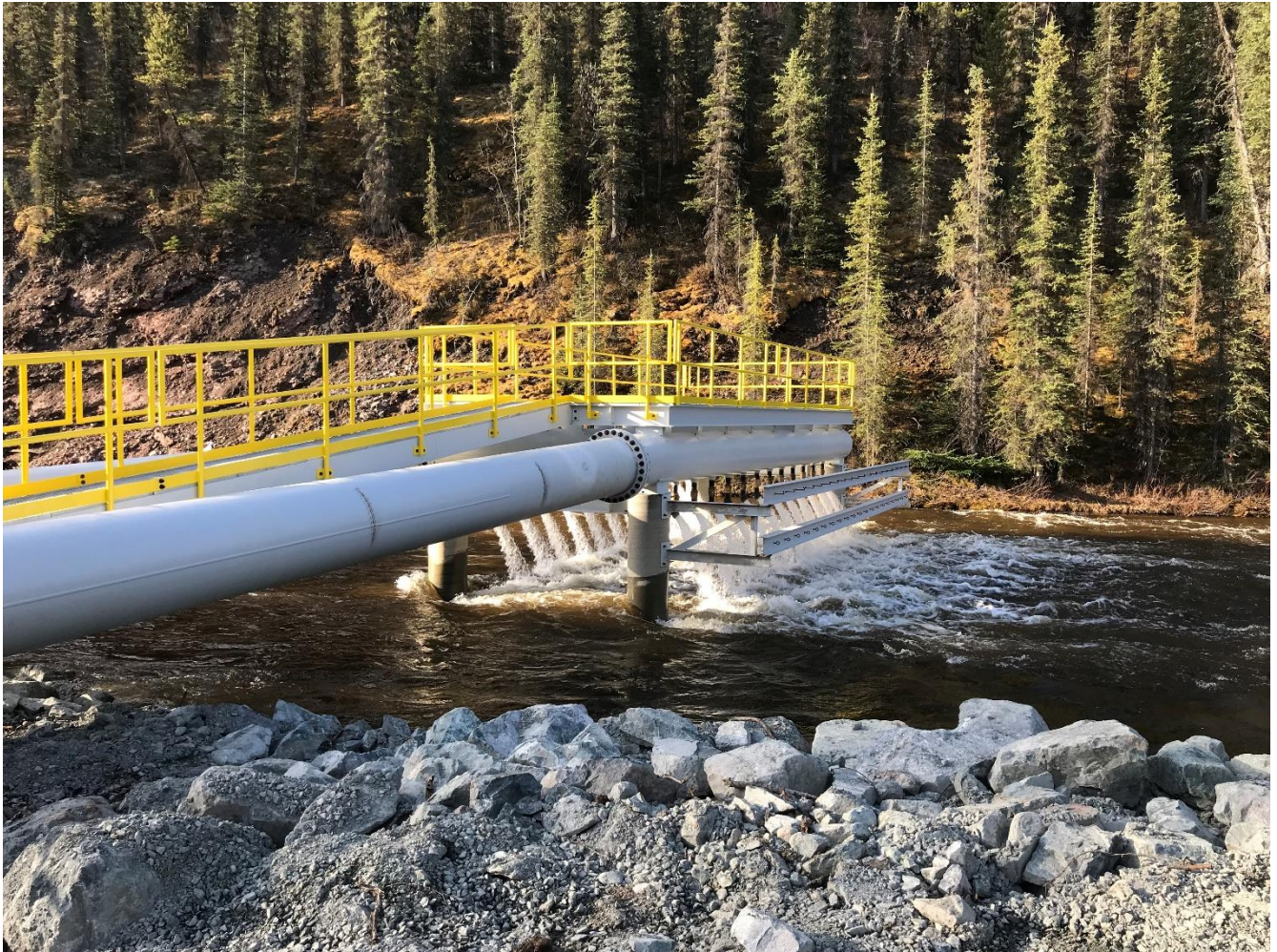
Plate 3.5-1: Attichika Creek Diffuser in operation.
