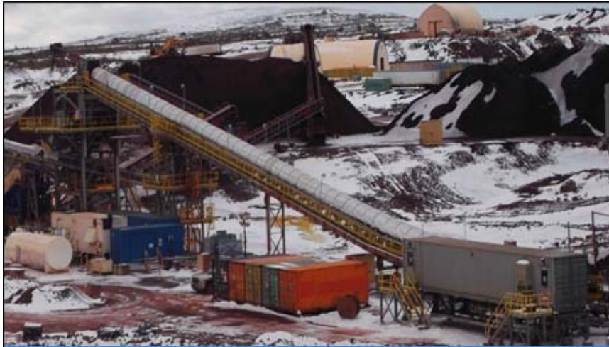
Sizing Stations & Dry Circuit Commissioned
