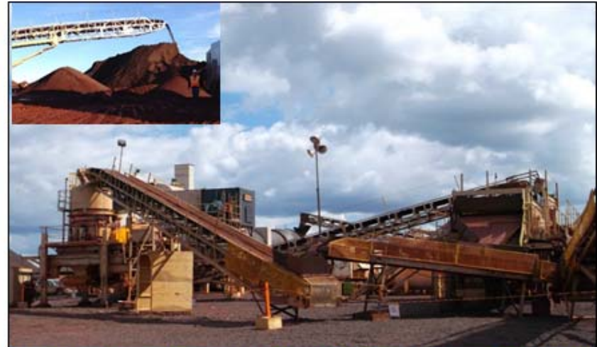
Mobile Crushing, Screening & Drying Commissioned
