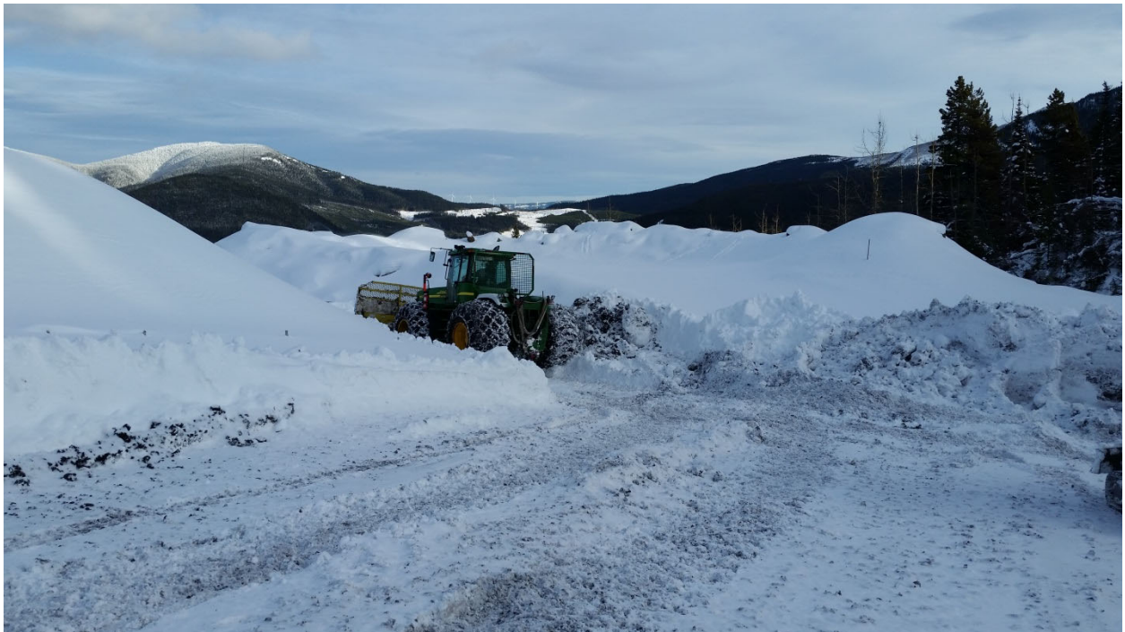
Photograph 1. Snowplow connected to a pickup truck and trailer with mini-excavator at the intersection of Chamberlain Road with the D-Road preparing for the last leg of the trip to the Chamberlain site. Photograph looking south-southwest. November 30, 2017.
