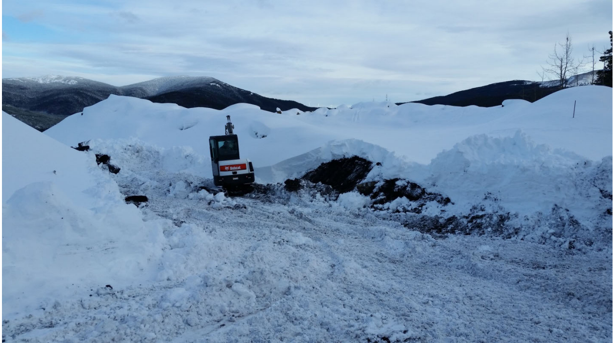
Photograph 3. Mini-excavator clearing snow from the waste rock pile prior to sample collection. Photograph looking east-northeast. November 30, 2017.
