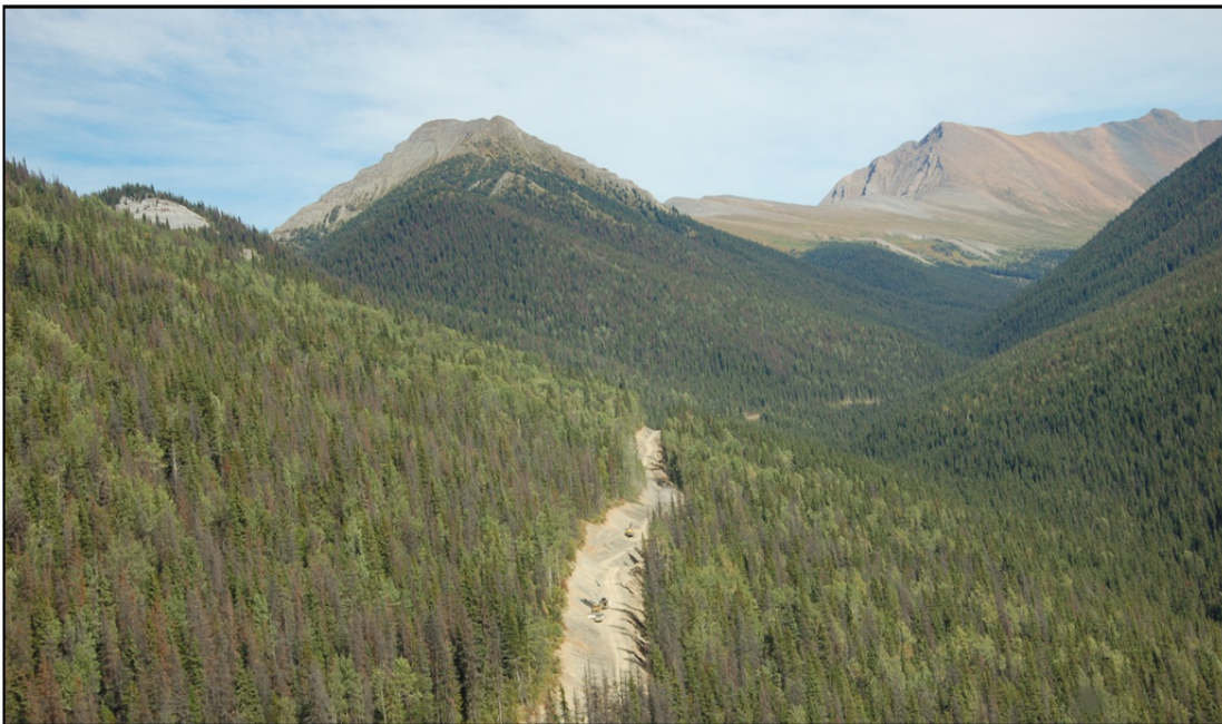
Photograph 3 – the site access road currently under construction. The road, constructed to support exploration activities, links into the existing forestry road network.
