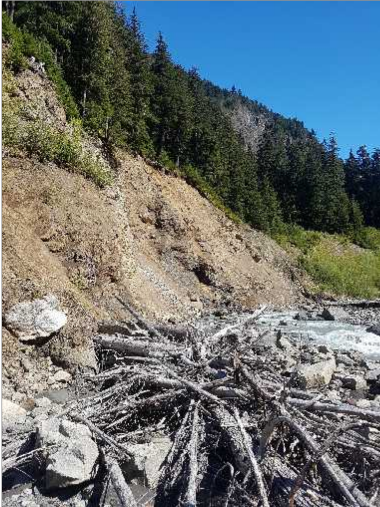
Figure 4: View of upstream section of road encroachment area. Date taken: 16-May-2017.
