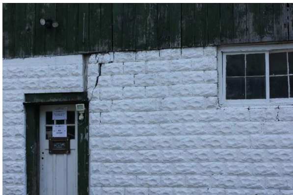
Plate 34: Localized cracking in the concrete foundation of the barn, looking west
