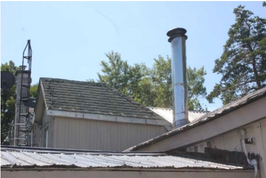
Plate 27: Shingled portions of roof in poor condition, looking southwest
