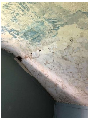
Plate 31: Cracking plaster on upstairs ceiling
