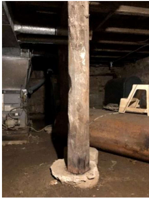
Plate 33: Support post on concrete footing in the basement showing signs of water intrusion
