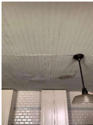
Plate 29: Water staining on kitchen ceiling from damage prior to roof repair
