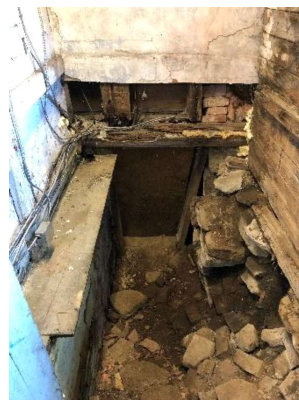
Plate 32: Cracking plaster, foundation shift and stairway obstruction on the basement staircase
