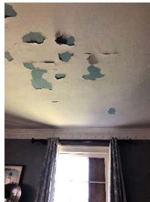
Plate 30: Localized plaster cracks and peeling paint in living room
