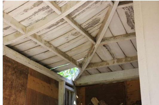
Plate 28: Gap in southwest corner of porch roof
