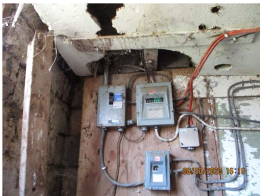
Plate 36: Electrical service equipment in the barn
