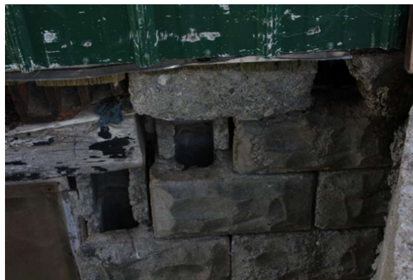
Plate 35: Broken blocks supporting rotting wooden lintels
