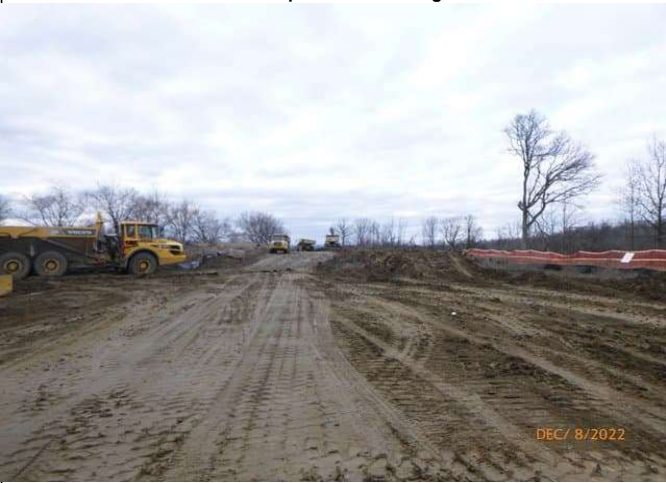
East Track Diversion - Cut to stockpile track profile South of Trib. A
