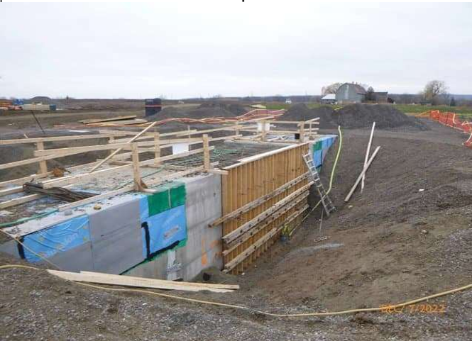
Box Culvert 2B - Exterior form work installation for cast in place section
