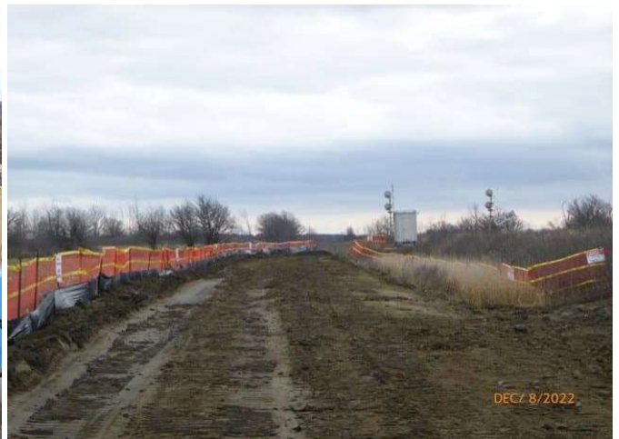
Track Realignment - Stripping topsoil for track realignment heading South to Ash Signals
