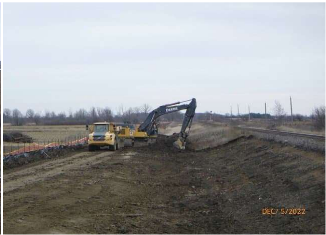
Track Realignment - Stripping topsoil for track realignment South of Sun Canadian track crossing
