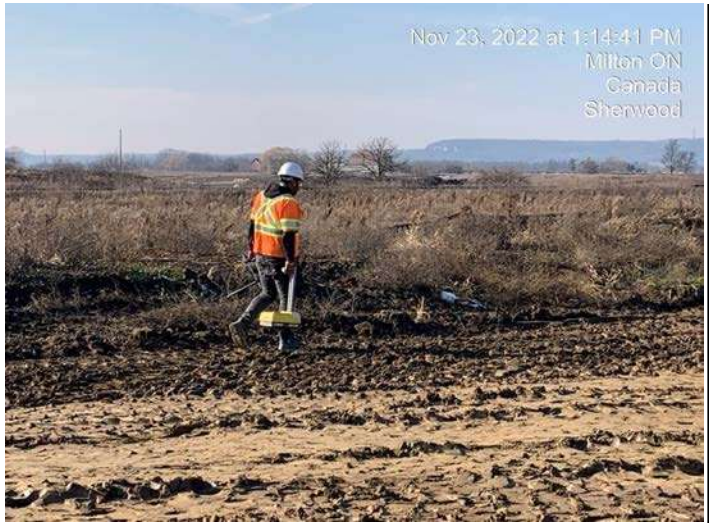
East Track Diversion - DCC QC Tech. conducting compaction testing on cut/fill material
