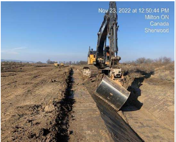
East Track Diversion - Excavation of material at east ditch for track diversion
