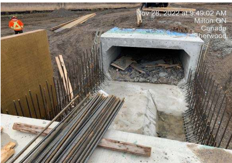
Trib A Cast-in-Place Culvert - Removal of form work as required at middle culvert section.
