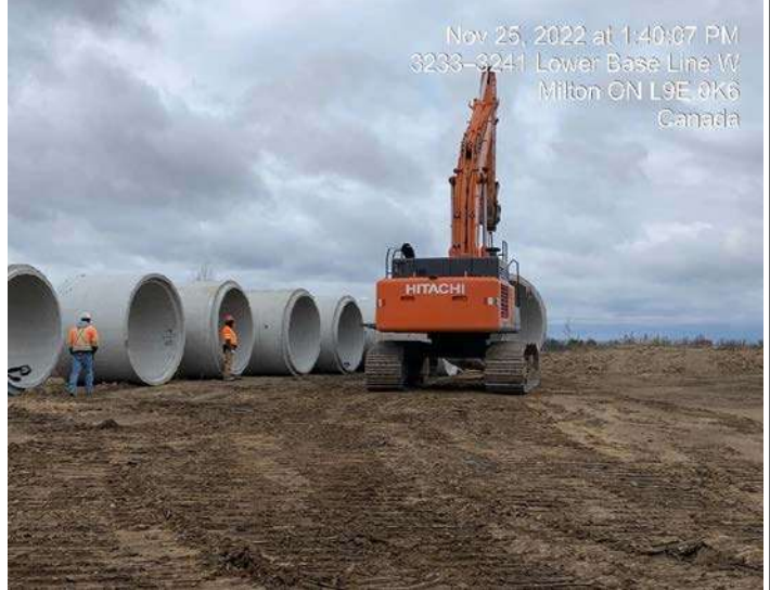
East Track Diversion - Move sewers from Laydown Area 1 to installation site area.
