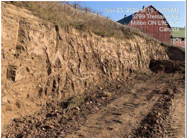
Pond 2 Area - Unsafe cut excavation at Riffle, embankment to be sloped
