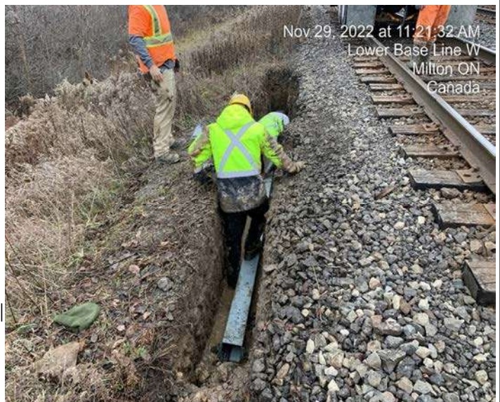
Lower Baseline Area - Encase signals in steel troughing at sewer crossing location
