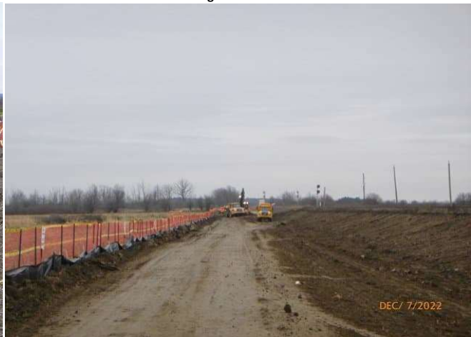
Track Realignment - Stripping topsoil for track realignment heading South to Ash Signals
