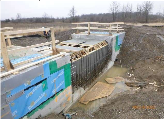
Box Culvert 2A - Interior form work installation for cast in place section
