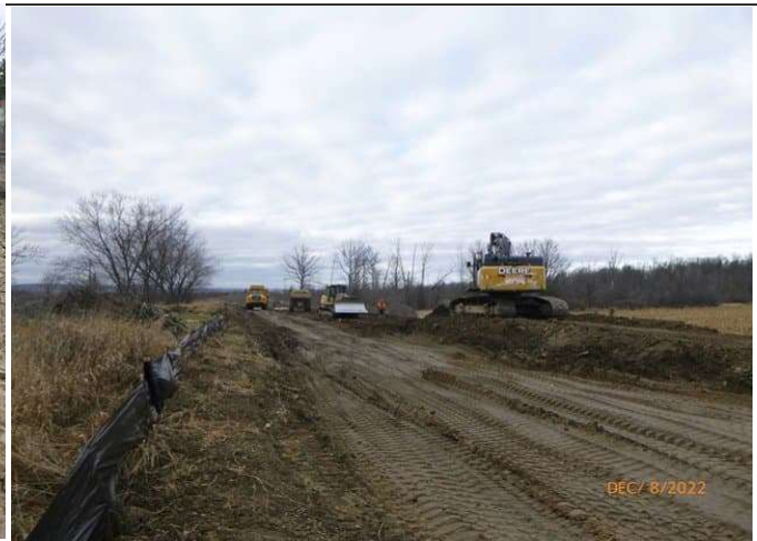
East Track Diversion - Cut to stockpile track profile South of Trib. A
