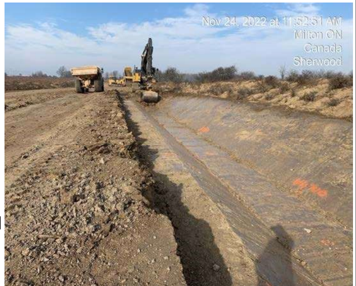
East Track Diversion - Excavation of material at east ditch for track diversion
