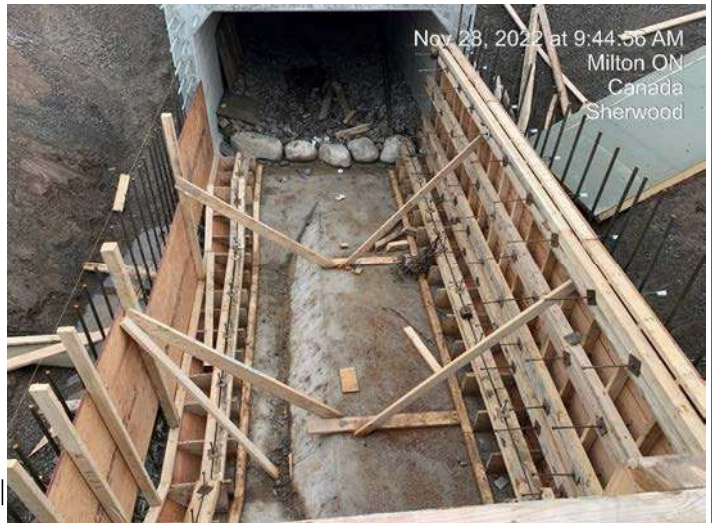
Trib A Cast-in-Place Culvert - Forming of inner walls and bracing for box culvert
