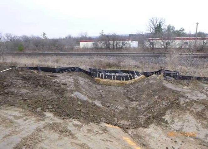
East Track Diversion - Installed ESC at West ditch outlet North of Culvert 3
