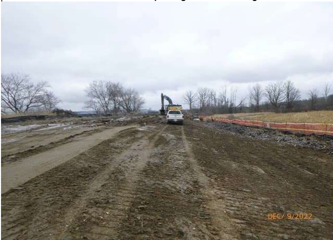
East Track Diversion - Cut to stockpile track profile South of Trib. A
