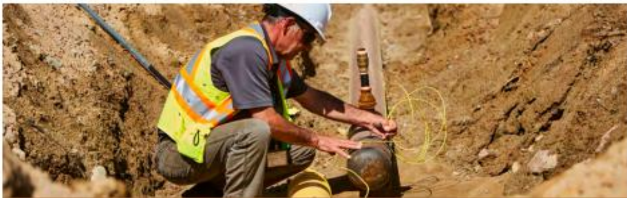
A CNL employee involved in converting the heating systems at the Chalk River Laboratories to natural gas, reducing site GHG emissions.
