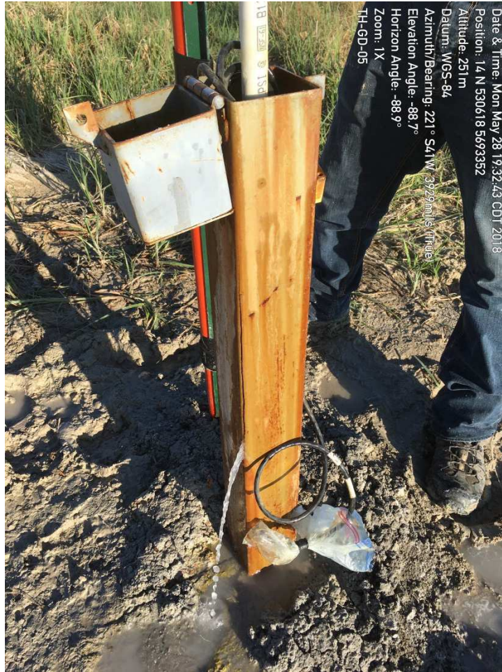
Figure 2: TH-GD-05 with a crack in the metal casing visible in the middle of the picture. Water leaked through after the PVC standpipe was opened, but stopped leaking after the PVC standpipe was re-sealed.
