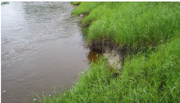
28+000: Erosion on left bank, looking upstream (2014).
