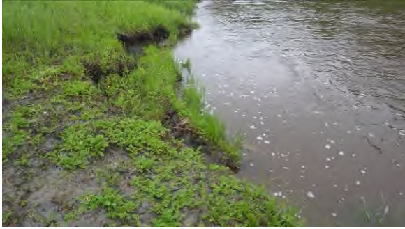
28+000: Erosion on left bank, looking downstream (2014).
