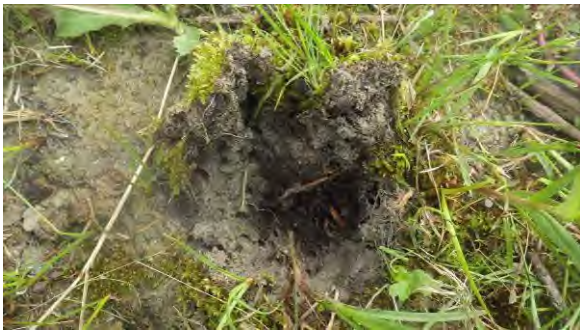
23+000: Silt deposition above organic soil on the left side of the creek in 2014.
