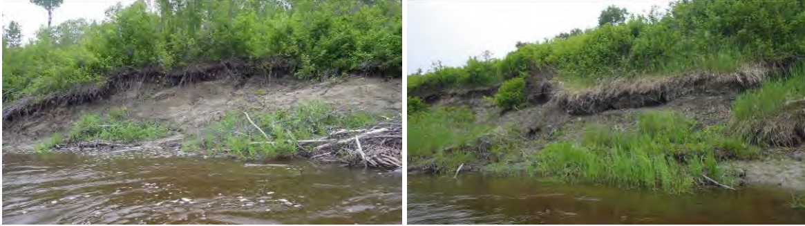
27+000: Eroded right bank approximately 100 m downstream (left) and 200 m downstream (right) from transect (2014 photos).
