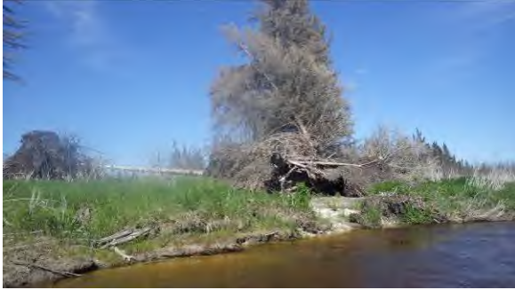
21+000: Erosion and fallen trees on left side of creek approximately 200 m upstream from transect 21+000 (2014).
