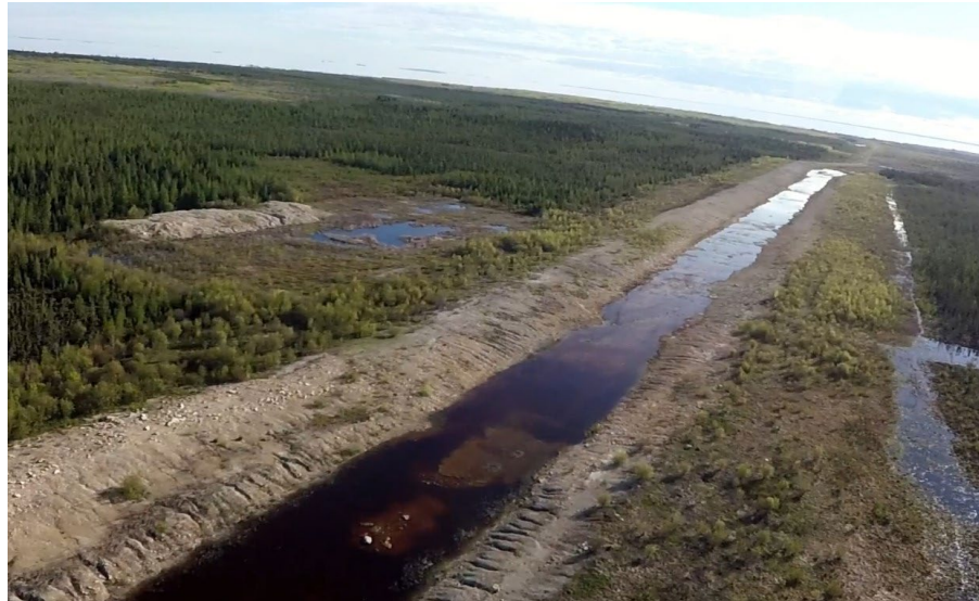
Figure 2 – June 2022 view of Reach 3 of the EOC, bedrock area, looking down channel. The temporary quarry site is in the upper left of the photo. A significant volume of water is stored in the channel at this time, draining from this reach of the channel over time. Note the high surface water levels adjacent to the channel. The metered flow contribution calculated at the down channel bedrock exposed area of Reach 3 was 0.18 M 3 /s at this time.
