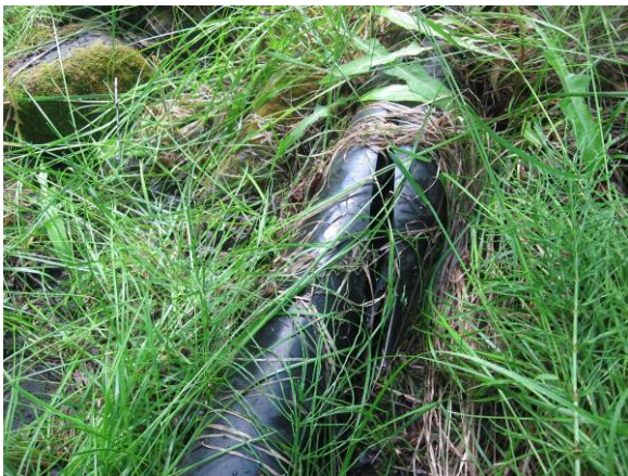
Photo 5. Broken water supply pipe
