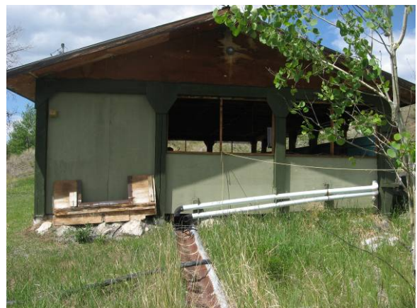
Photo 30. Hatchery discharge pipe outside building
