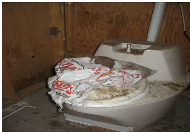
Photo 35. Composting toilet inside hatchery building
