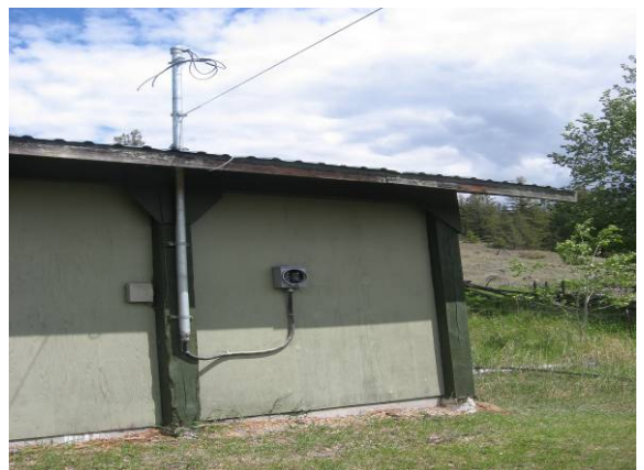
Photo 36. Disconnected electrical service
