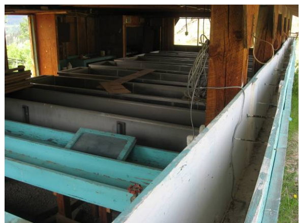
Photo 18. Water supply wood header box (interior) plus troughs
