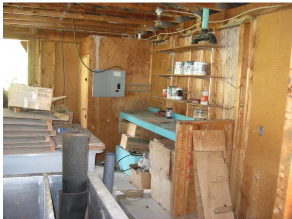
Photo 33. Workbench and electrical service panel
