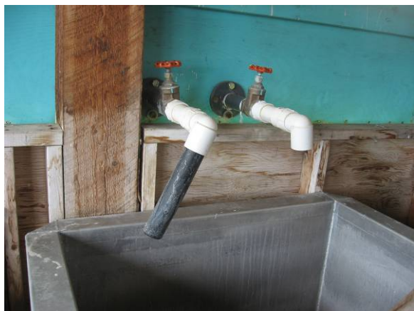
Photo 21. Water supply valves to troughs
