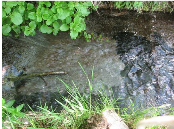
Photo 4. Damaged water intake box
