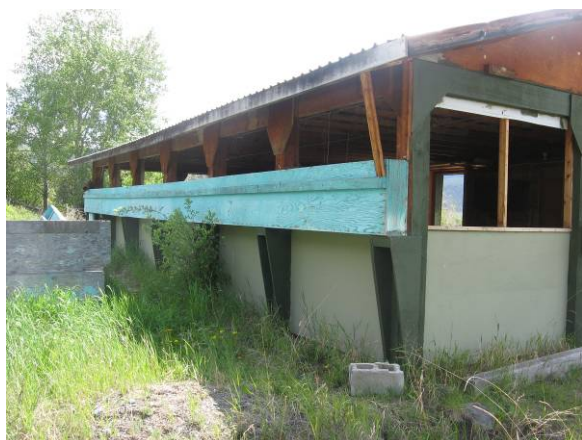
Photo 17. Water supply wood header box (exterior)
