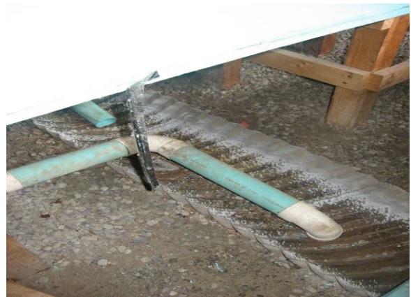
Photo 28. Discharge pipe at trough outlet
