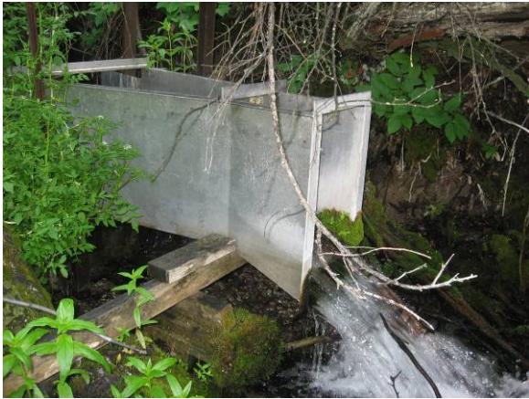
Photo 3. Spring waterflow measurement weir
