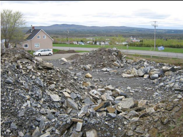
Photograph 3: Bare ground and piles of earth materials on the site planned for the reservoir and the drinking water treatment facility; looking east (May 2007).
