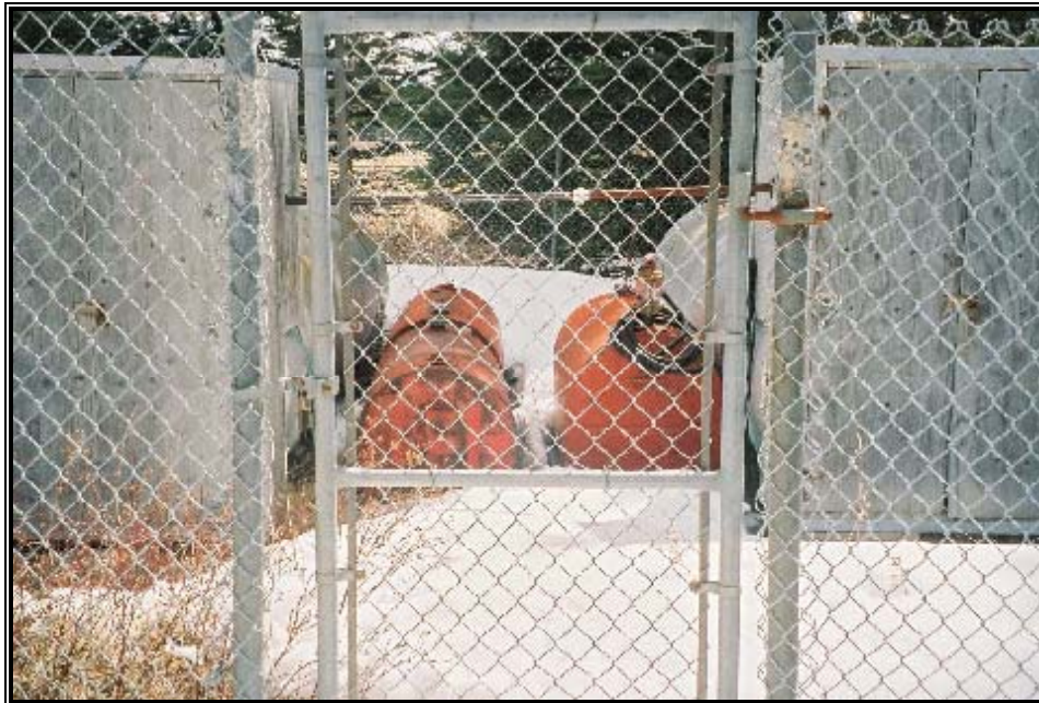
Photo 3. Aboveground storage tank and fuelling facilities
