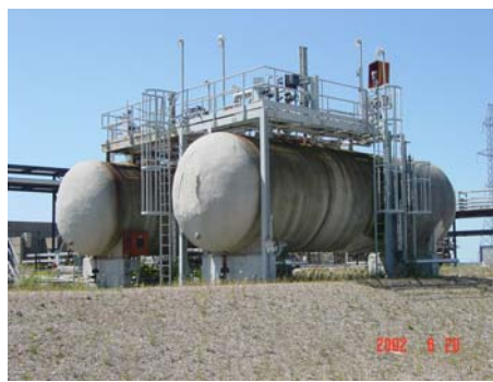
Photo 8 – Propane Storage Area
