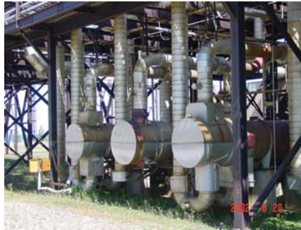
Photo 11 - Process Effluent/Process Feed Water Heat Exchangers
