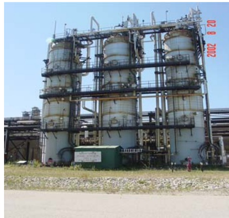
Photo 6 – Plant B Degasser Tower
